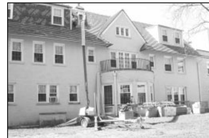
A single man-lift was used to install siding to third floor dormers.
